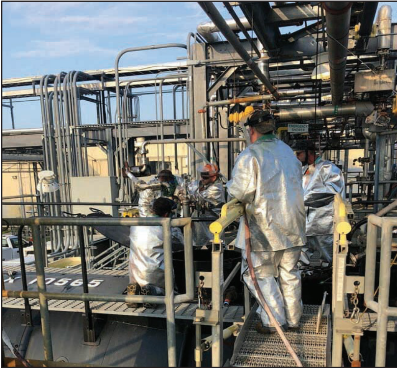
Multiple divisions of Pine Bluff Arsenal's Directorate of Public Works, including the Pipe Shop and Fire Department, Directorate of Ammunition Operations and Directorate of Risk Management and Regulatory Affairs-Safety Division connect a railcar to the Arsenal's white phosphorus system for unloading. The system must be kept in water to prevent catching fire.
