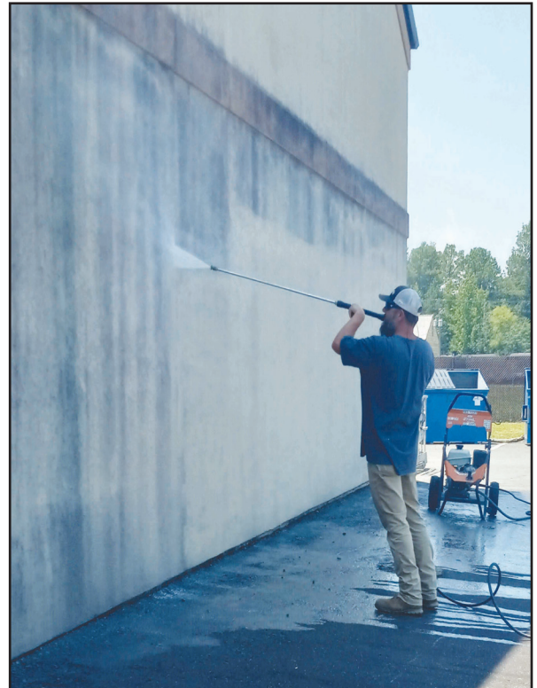
Jeff Daigle with Pine Bluff Arsenal's Directorate of Public Works Carpenter Shop power washes a building. U.S. ARMY PHOTOS BY TRACEE MILLS-BOID-DPW
