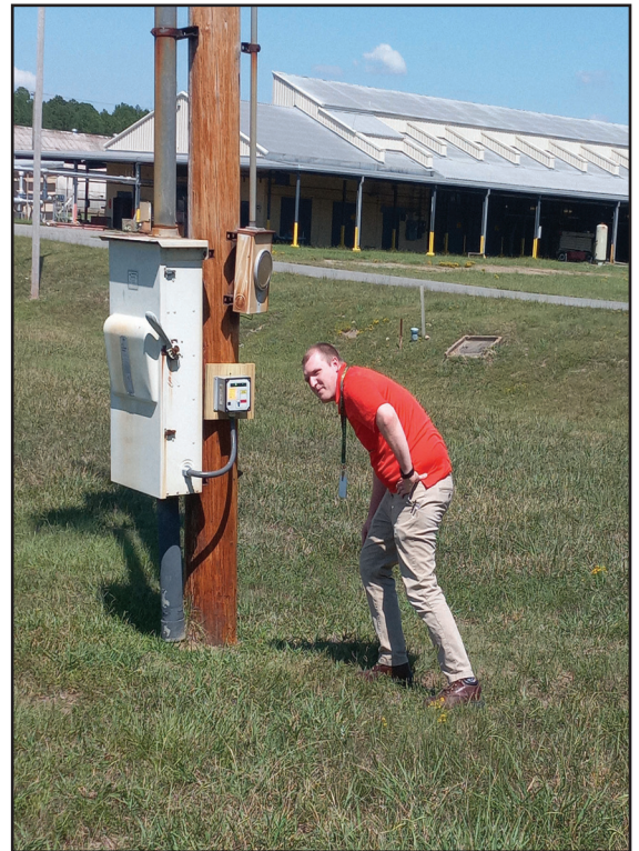
Davis Harp with Pine Bluff Arsenal's Directorate of Public Works-Engineering, Plans and Services Division, verifies surge protection installations on the Arsenal.
