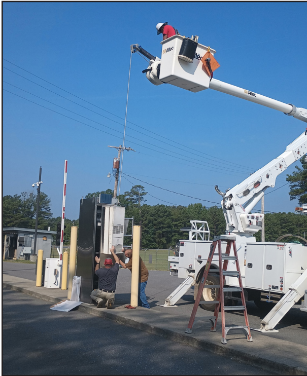
Photo above left, Pine Bluff Arsenal's Directorate of Public Works Electric Shop personnel James (Steven) Smith (in bucket), Jesus (JR) Rodriguez, left, and Brad Rauls, right, install a new air conditioner for a camera kiosk.
