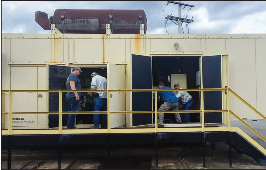
Pine Bluff Arsenal Instrument Shop personnel perform routine maintenance on a generator at the white phosphorus production facility. Pictured from left are Drue Owen, Terry Coffman, Jerry Arledge and Mike Hancock. U.S. ARMY PHOTOS BY TRACEE MILLS
