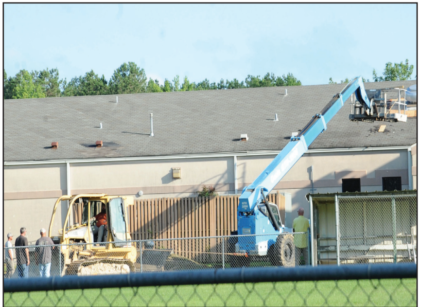
Pine Bluff Arsenal Directorate of Public Works personnel work on the roof at the Creasy Complex during a hot day in July. U.S. ARMY PHOTO BY HUGH MORGAN
