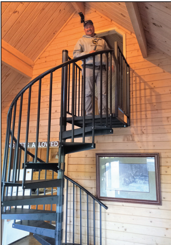
Daniel Edwards with Pine Bluff Arsenal's Directorate of Public Works Carpenter Shop applies the finishing touches to the spiral staircase build for the Cabin in the Woods on Tulley Lake.
