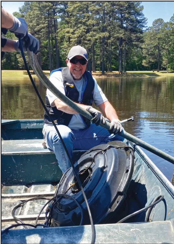
William (Bill) Dean with Pine Bluff Arsenal's Directorate of Public Works Electric Shop repairs an aerator at the Conference Center on Dilly Pond.
