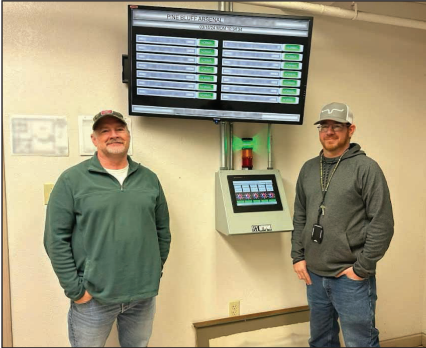
Donny Pumphrey, Electric, HVAC, and High Voltage Supervisor, and Ryan Saunders show a new system to facilitate the modernization of utility air and steam systems. Pine Bluff Arsenal's Directorate of Public Works, Operations and Maintenance Division, is in the process of developing a control system giving real time run and alarm status. In turn, this will assist the O&M team to monitor all air compressors and steam boilers providing support for Ammunition Operations. This monitoring will speed up response time to issues of equipment and reduce production downtime. The control system was developed by Saunders. U.S. ARMY PHOTO BY CAITLIN THOMAS, PBA DPW
