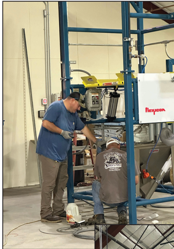
Wes Hoffman and Shawn Eversole, with Pine Bluff Arsenal's Directorate of Public Works, works to install new equipment and electrical systems at an Arsenal building.
