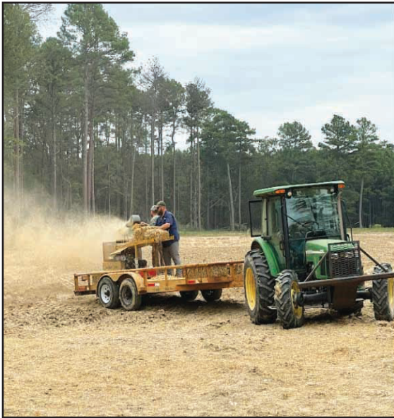
Keith Stanley, Clayton Smith and Robert Morrison with Pine Bluff Arsenal's Directorate of Public Works work together to seed and blow straw over the first and second completed sections of a sewer project.
